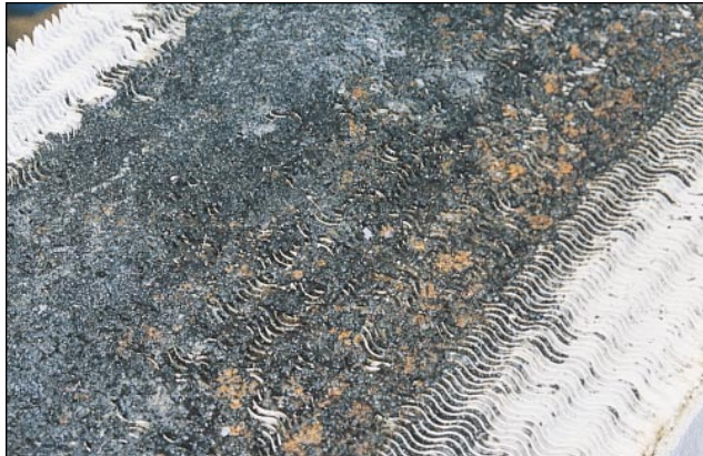
Full-strength coil cleaner applied to the surface of cooling coils then flushed with high-pressure hot water will result in a coil that appears to be clean, but may actually be a hotbed for microbial growth. Increased pressure drop and reduced air volume through such coils is a red flag that says it's time for a replacement.
