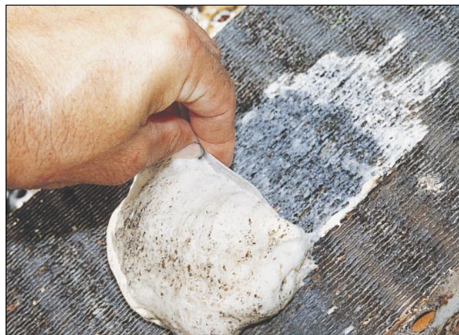
If properly maintained and regularly cleaned with coil cleaners and hot water, a coil's interior as well as its exterior can be kept clean. The bubbling action of foaming cleaners can actually lift the dirt from the coil's interior.
